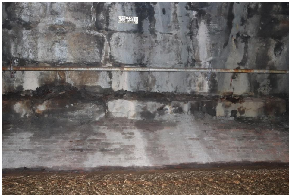
Photo 12: View within tunnel north of the recessed platform, detail of invert, looking east
