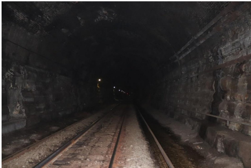
Photo 10: View within tunnel, looking north from northern end of the southern cut-and-cover section towards the bored section
