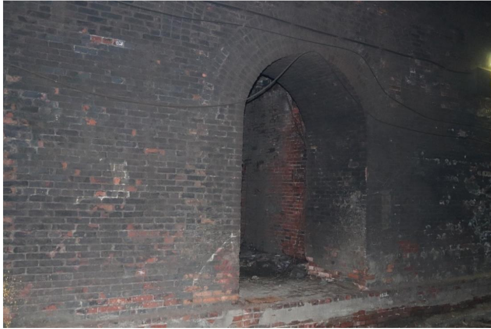
Photo 11: View within tunnel, detail of recessed platform near West Lombard Street, looking southeast
