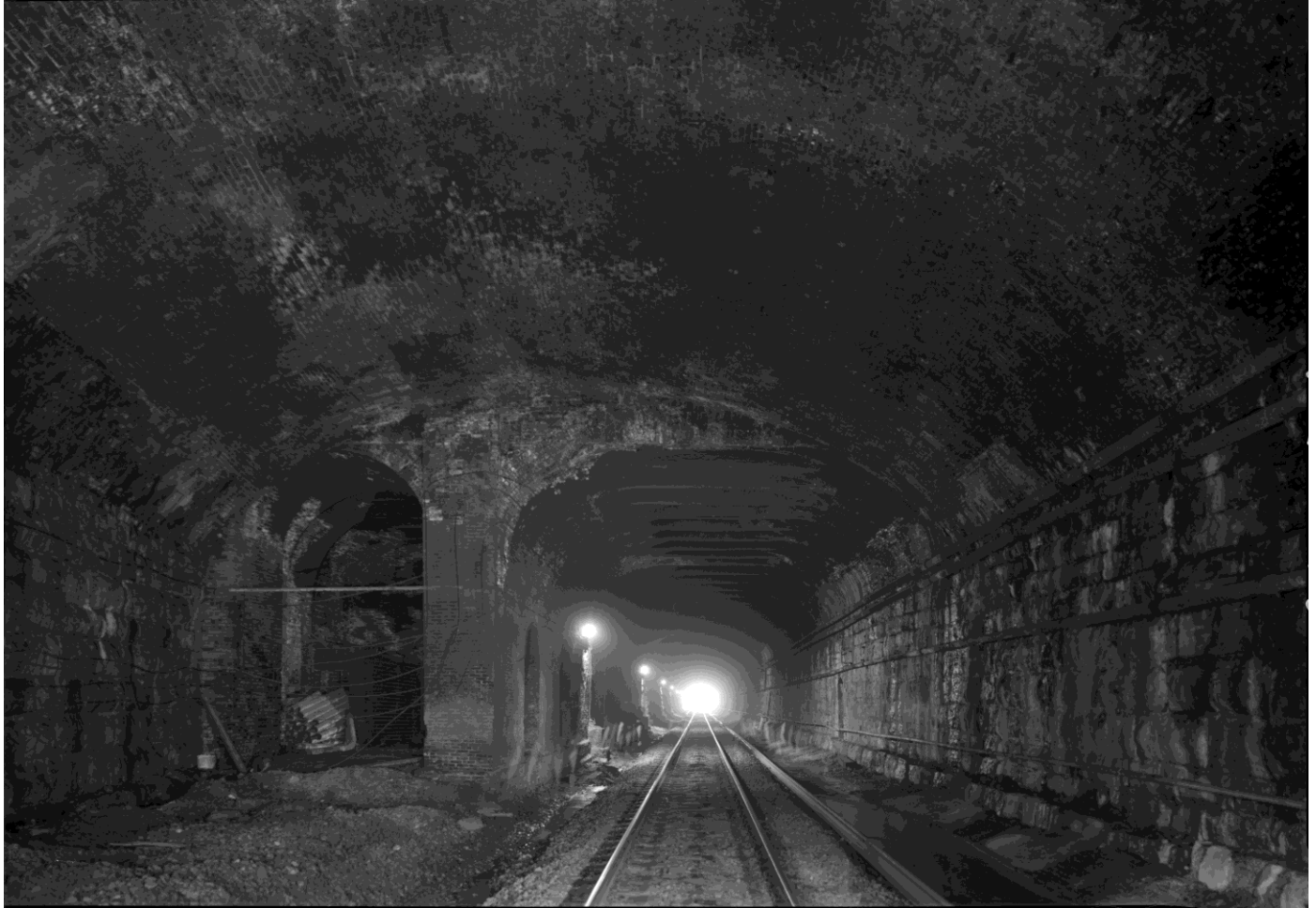
Figure 2: The arched opening east (left) of the tracks leading to the incomplete underground platform, and the original steel girders running east-west across the tops of the arches above the railroad tracks, looking south, 2021.
