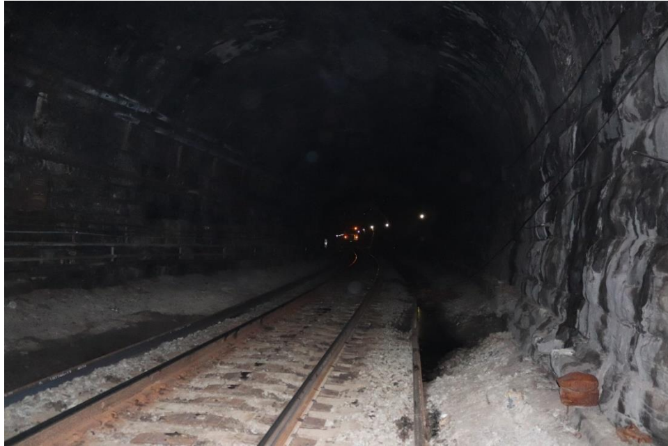
Photo 13: View within tunnel, looking north from the original south portal to the southern cut-and-cover section
