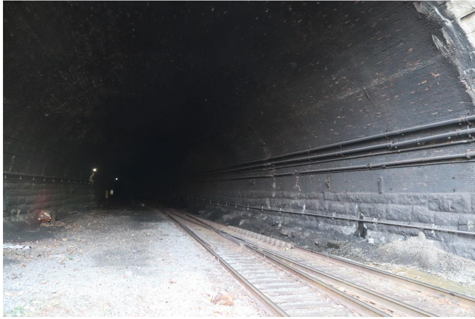
Photo 5: Tunnel interior, looking southwest from the north portal to the northern cut-and-cover section
