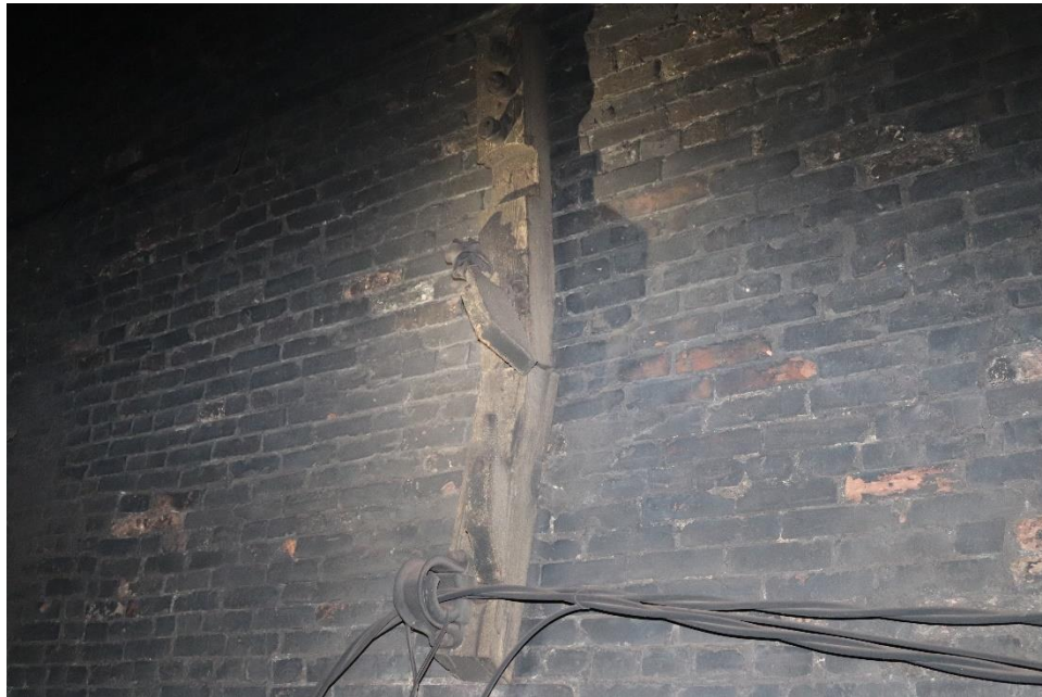
Photo 8: Typical original wood block for holding electrical wires and lighting, looking east near Mount Royal Station
