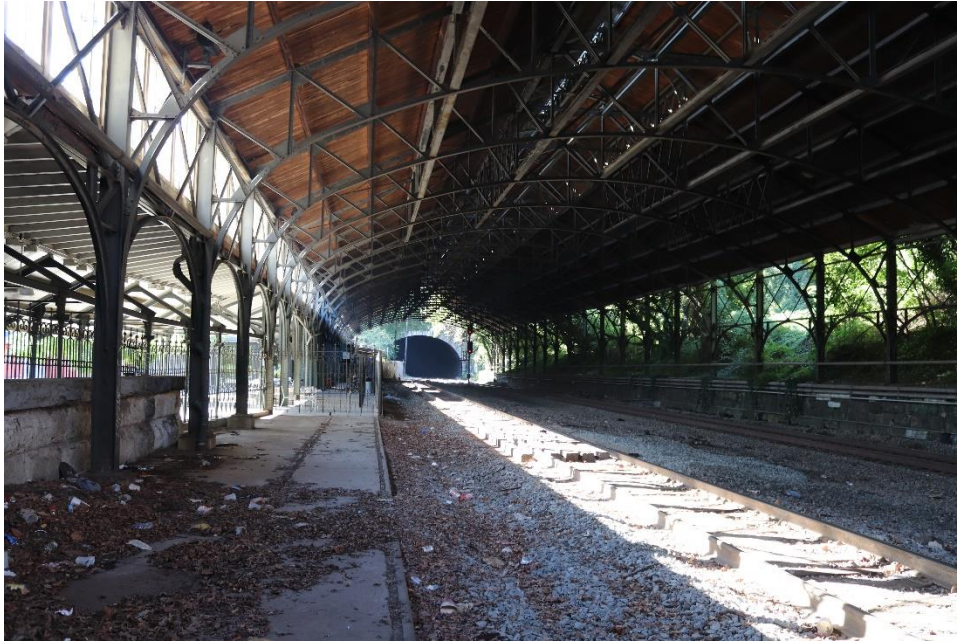
Photo 1: Inside the trainshed at Mount Royal Station, looking southwest at the north portal
