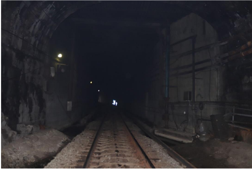
Photo 15: View within tunnel, looking south from the 1895 south portal to the boxed concrete section
