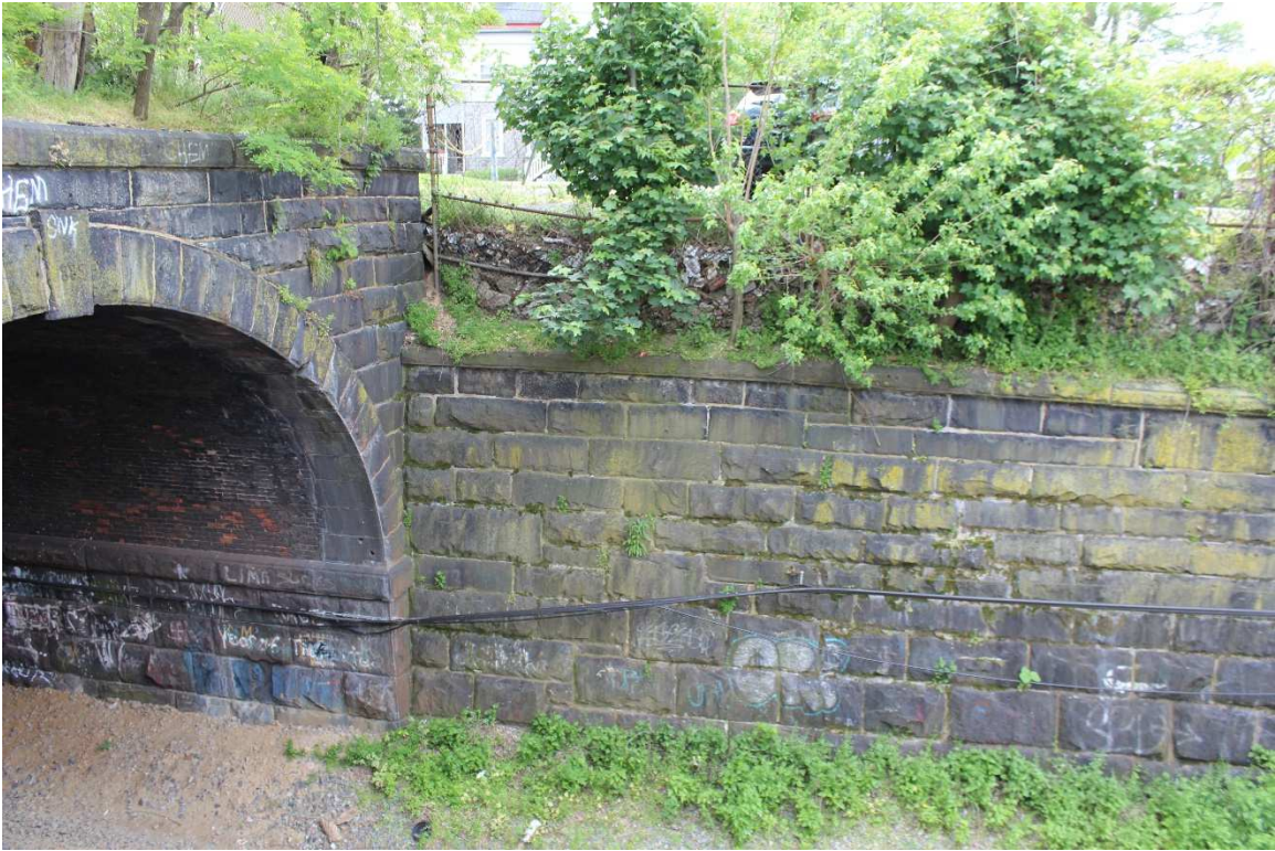
Photograph #3: Boone Tunnel northeast portal and north retaining wall, looking north. May 20, 2020.
