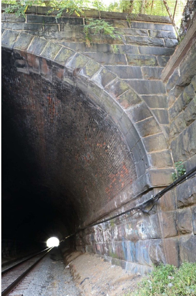
Photograph #9: Boone Tunnel southwest portal and interior, looking northeast along south wall. October 15, 2021.
