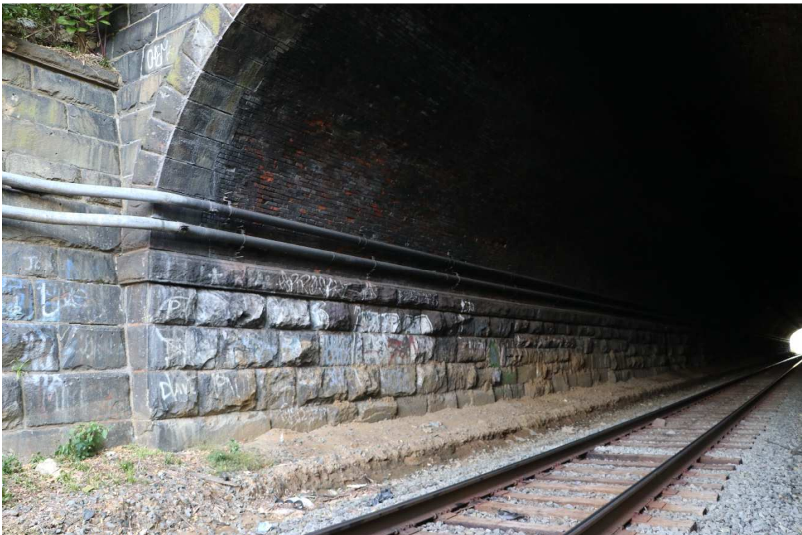
Photograph #8: Boone Tunnel southwest portal and interior north wall, looking north. October 15, 2021.
