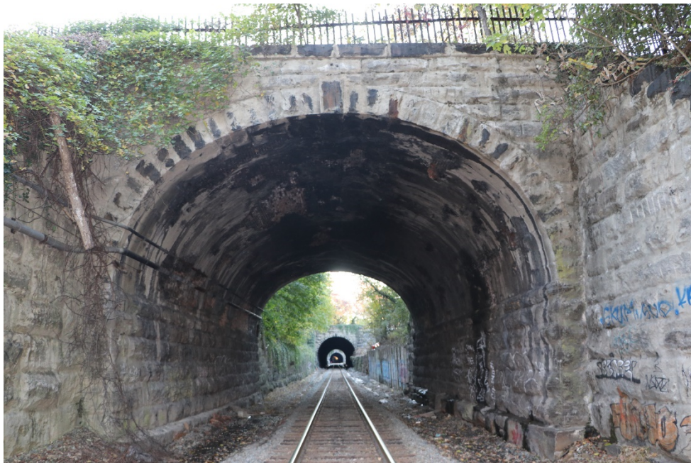
Photo 3: Detail of east portal and tunnel interior, looking west to Calvert Street
